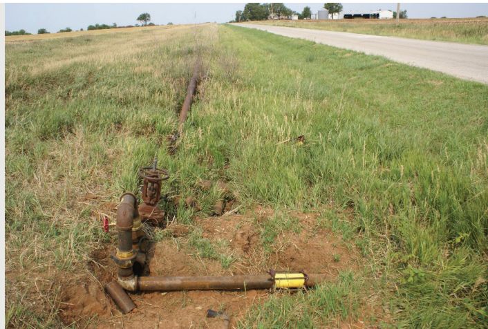
FIGURE 1. Private lines are not always installed to normal standards.
